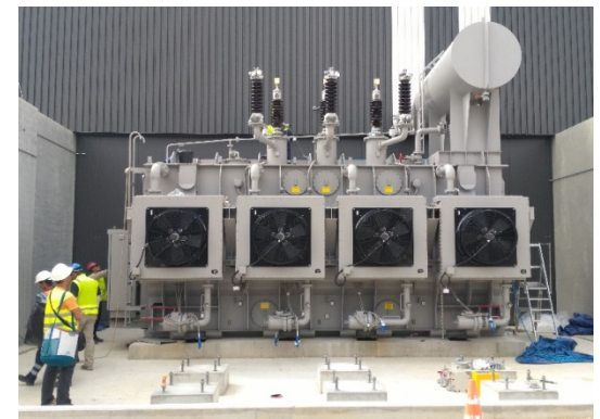
< Bldg. 32, CS Transformer >
