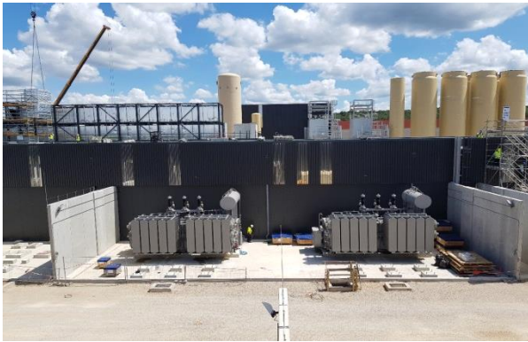
< Bldg. 33, VS1 Transformer >
