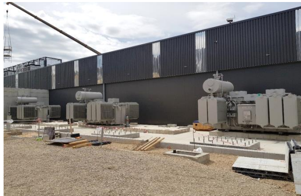
< Bldg. 33, CCS Transformer >
