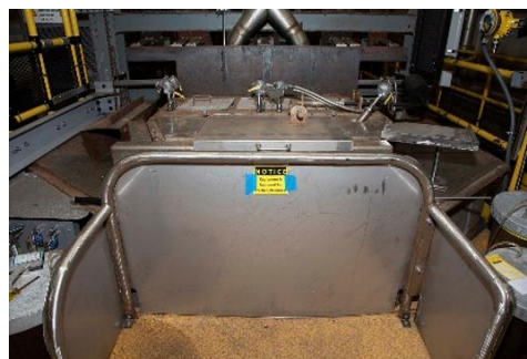
Restored electrolytic cell at Y-12
